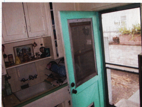
The way the old kitchen door was installed affected countertop and cabinet placement.
